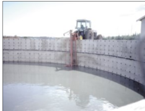
Figure 3.7. Liquid manure storage - circular concrete tank.
